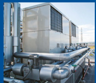
Emergency-ready Gas cogeneration
