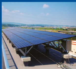
Solar power generation panel
