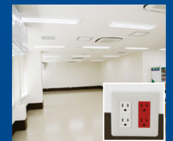
Power outage shelter area (3rd floor) (Red power outlet can be used even during power outage)
