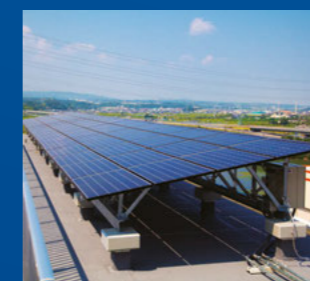
Solar power generation panel
