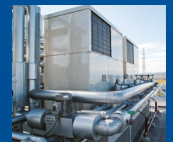
Emergency-ready Gas cogeneration
