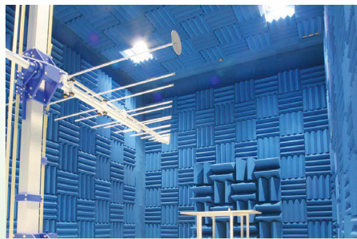
RF Anechoic Chamber
