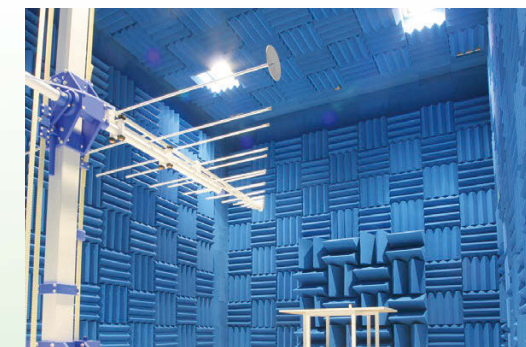
RF Anechoic Chamber
